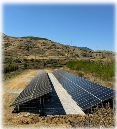
8. Panelet Diellore - Solar Panels
